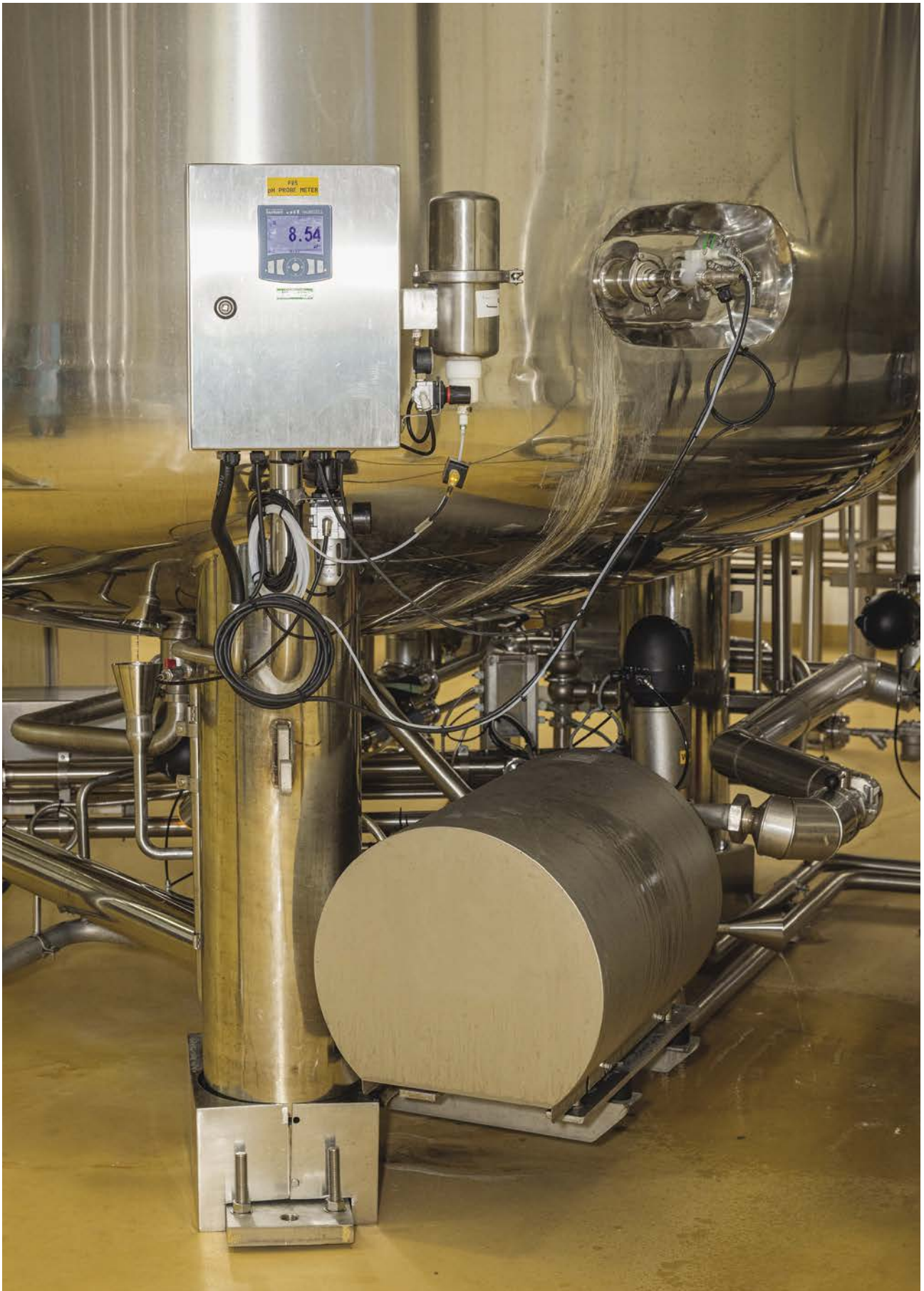
pH monitoring on fermentation tank
