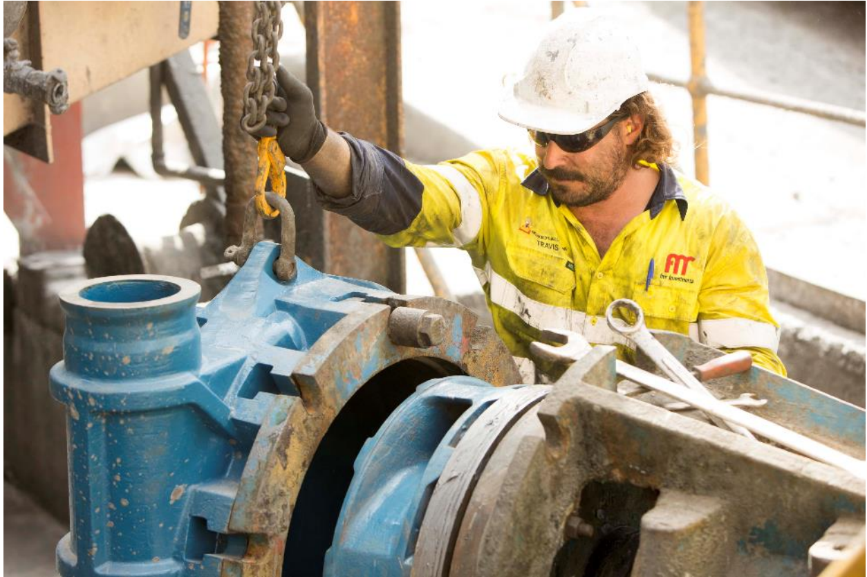
Figure 1 Regular inspections and maintenance help ensure both duty and standby mill discharge pumps are ready for action (IMG: _30A9200.jpg)
