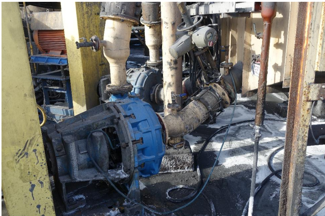
Figure 3: Duty and standby pumps always allow for a backup option (IMG:DSC00797.JPG)
